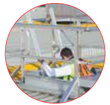
RETRACTABLE STILES FOR SAFE ACCESS THROUGH ROOF HATCH
